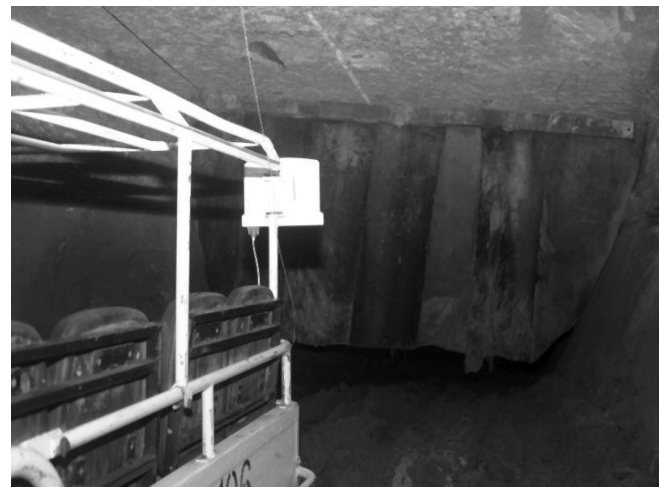
Fig. 12. Rubber curtain to control air circulation
