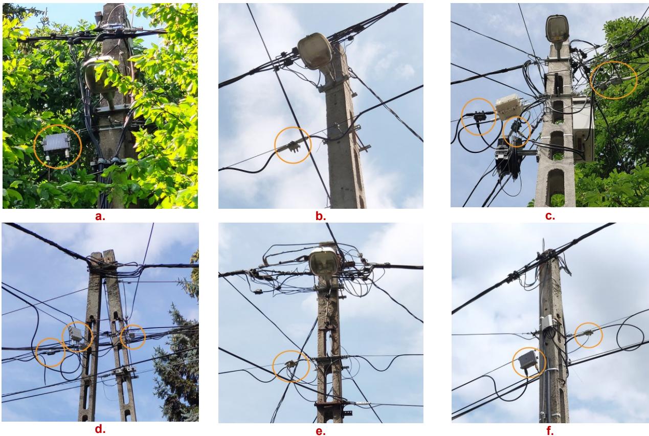
Fig. 7. Potential leakage sources of measurement samples; they are denoted by orange circles and are also listed in Table III
