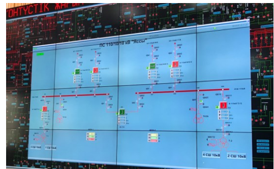
Fig.6. Dispatching control of the substation of the power system in SCADA
